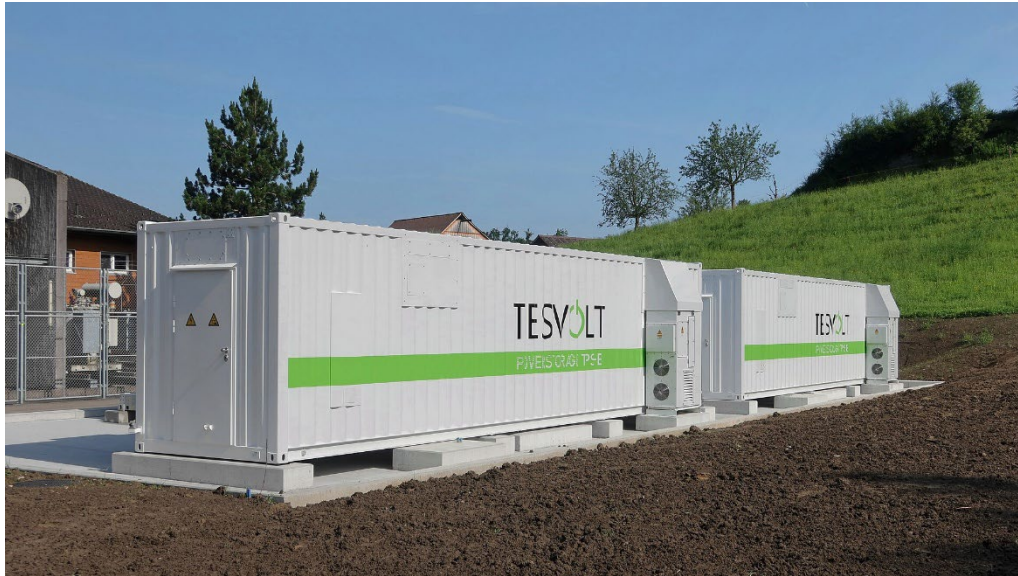
Figure 9: A large battery storage power station with a capacity of 6.24 MWh and an output of 5 megawatts (Tevolt TPS-E). Source: Wikimedia (2024)
