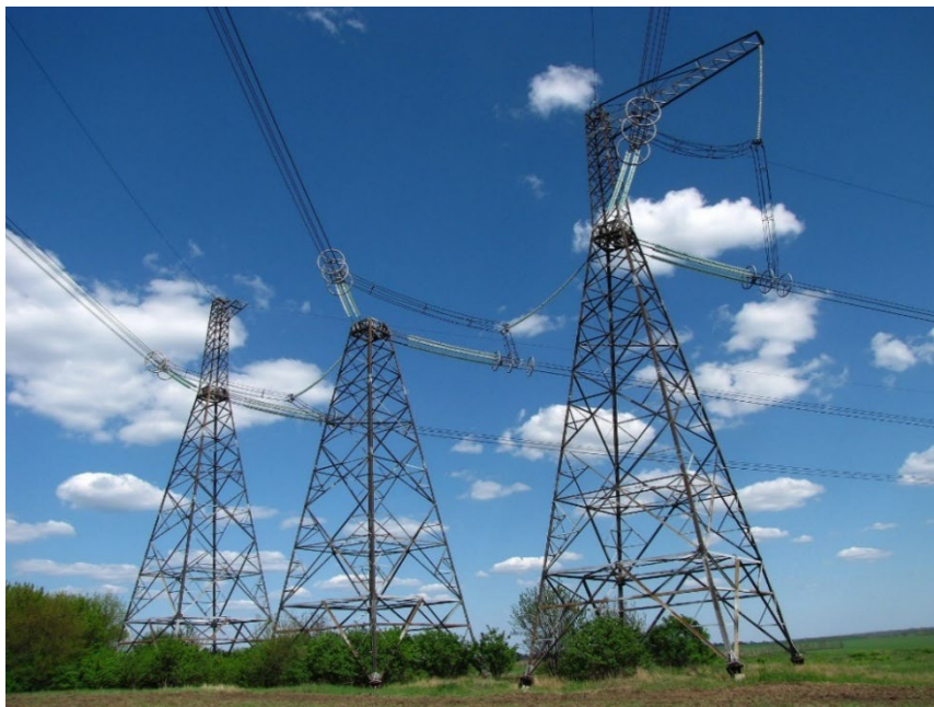
Figure 5: Anchor pylon of high-voltage overhead power line 750 kV. Source: Dimtryi Novoklimov (2010),
