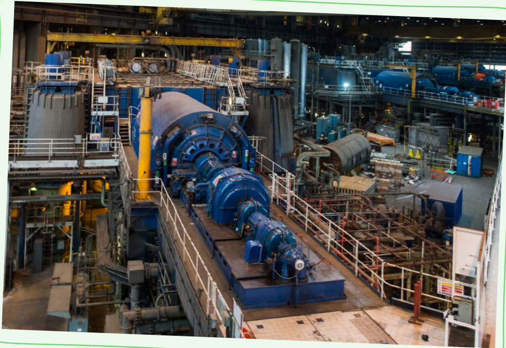
The turbine hall at Drax Power Station
